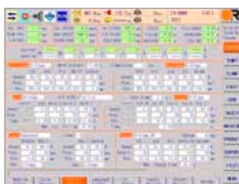
Overall setting screen
